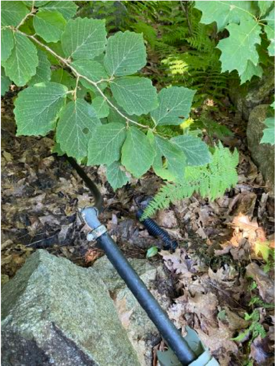
Fig. 9 - Gray Water Draining from Gray Water Discharge
