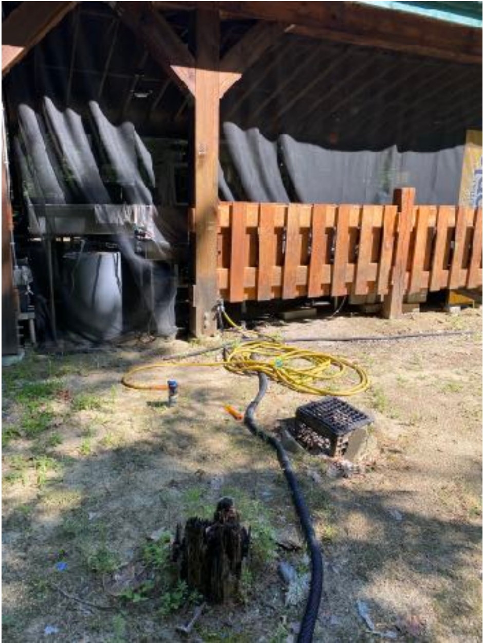
Fig. 7 - Gray Water Line from Kitchen Sink
