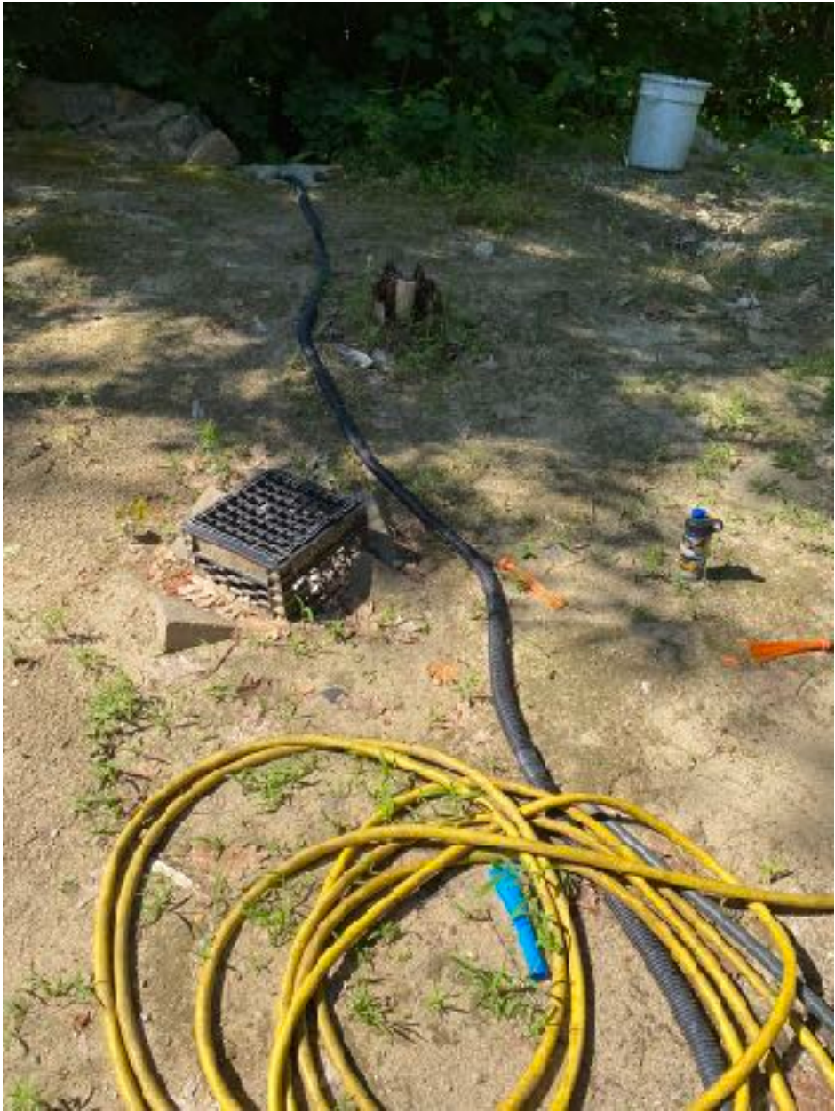
Fig. 6 - Gray Water Line
