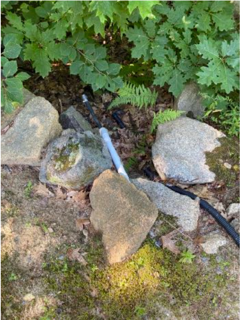
Fig. 5 - Gray Water Discharge and Water Supply
