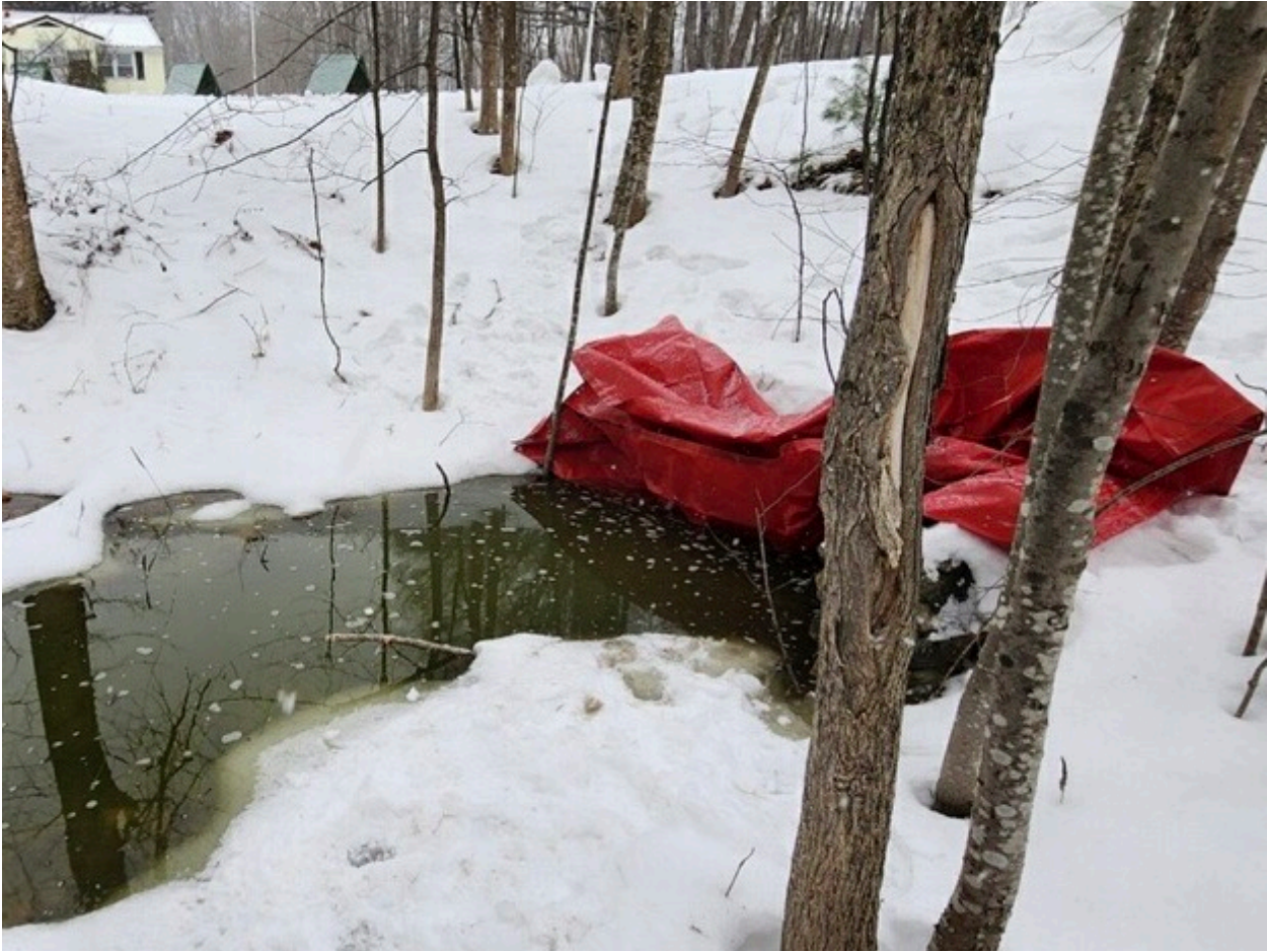
Fig. 4 - Green, cloudy fluid moving toward culvert under the driveway of 183 Whittier Highway. Culvert has been diked with red salvage cover - 01/16/2024
