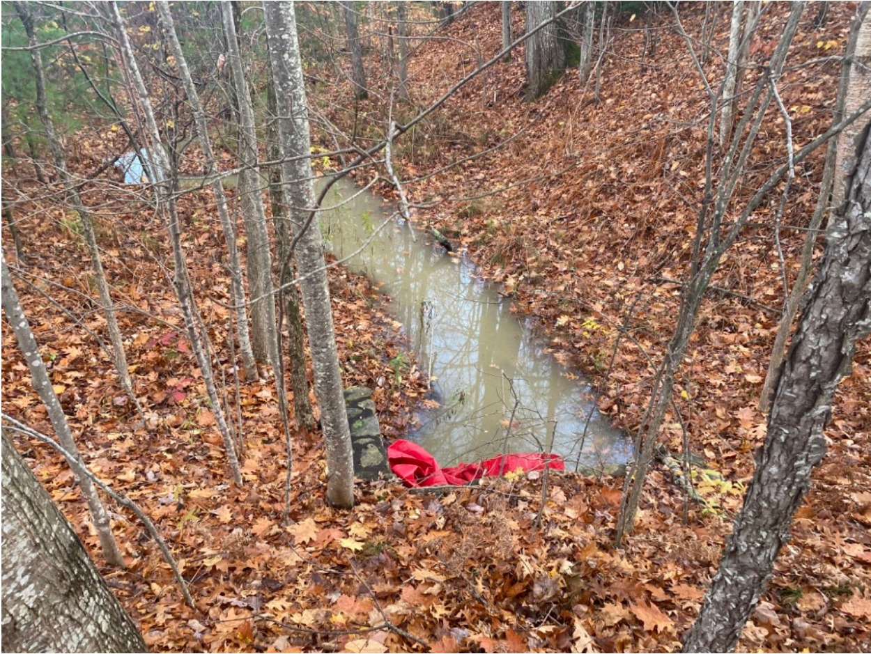
Fig. 4- Clay-colored fluid moving toward culvert under the driveway of 183 Whittier Highway. Culvert has been diked with red salvage cover - 11/10/2023
