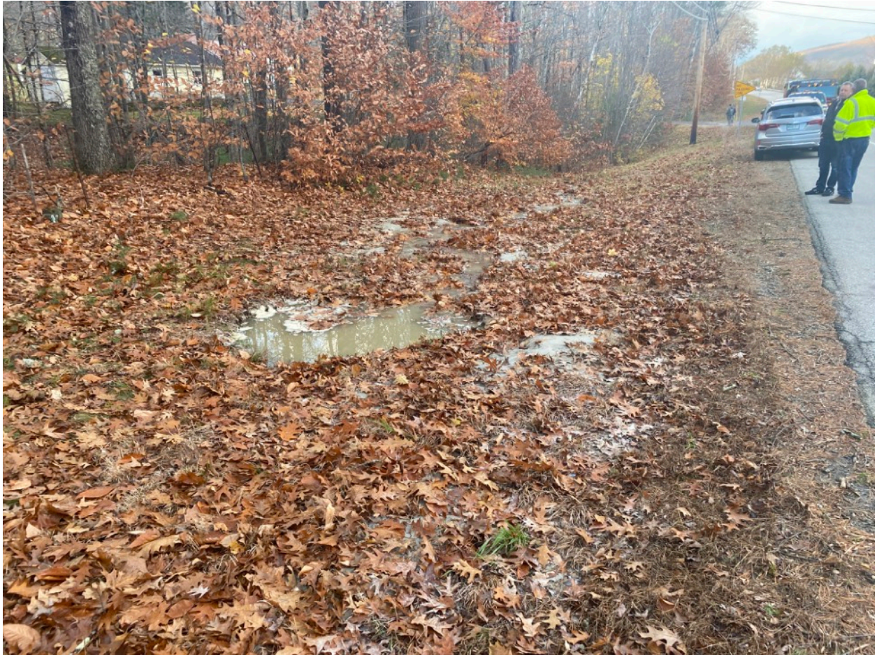
Fig. 1 - Clay-colored fluid collecting in and flowing out of an approximately 3 foot diameter hole and downhill in front of 183 Whittier Highway - 11/10/2023
