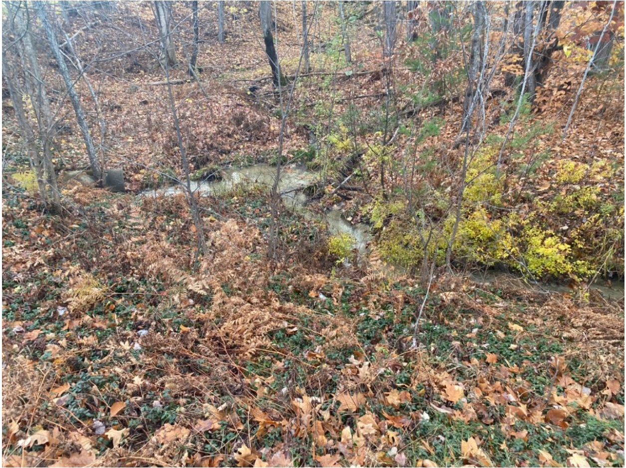
Fig. 5 - Clay-colored fluid moving through culvert under the driveway of 183 Whittier Highway (left side of image) - 11/10/2023
