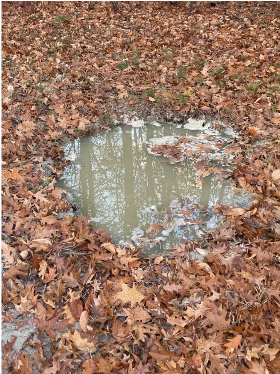
Fig. 2 - Clay-colored fluid collecting in and flowing out of an approximately 3 foot diameter hole in front of 183 Whittier Highway. Additional sediment is noted in an approximately 6 foot diameter area around the hole - 11/10/2023
