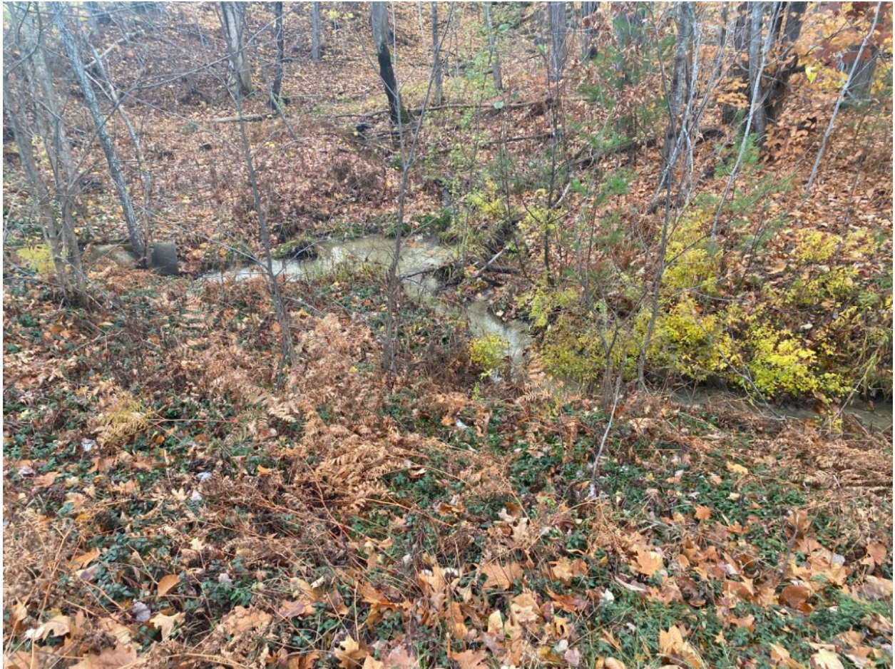
Fig. 5 - Clay-colored fluid moving through culvert under the driveway of 183 Whittier Highway (left side of image) - 11/10/2023
