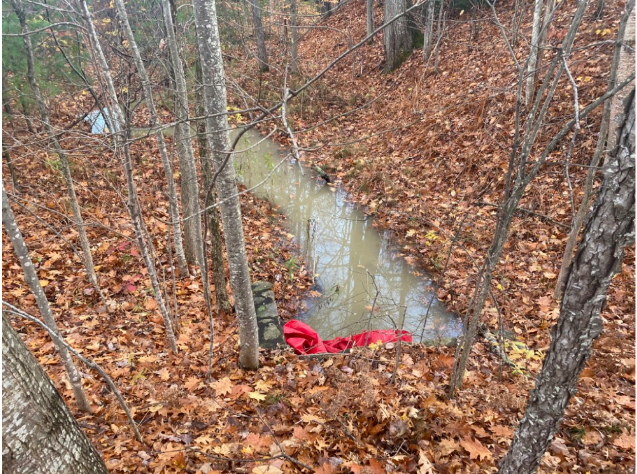
Fig. 4- Clay-colored fluid moving toward culvert under the driveway of 183 Whittier Highway. Culvert has been diked with red salvage cover - 11/10/2023
