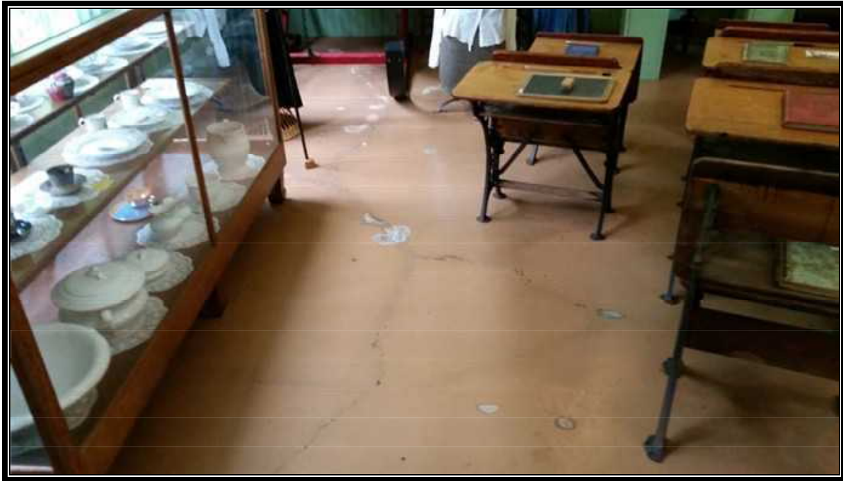
Photo 5: Cracks in floor slab.
