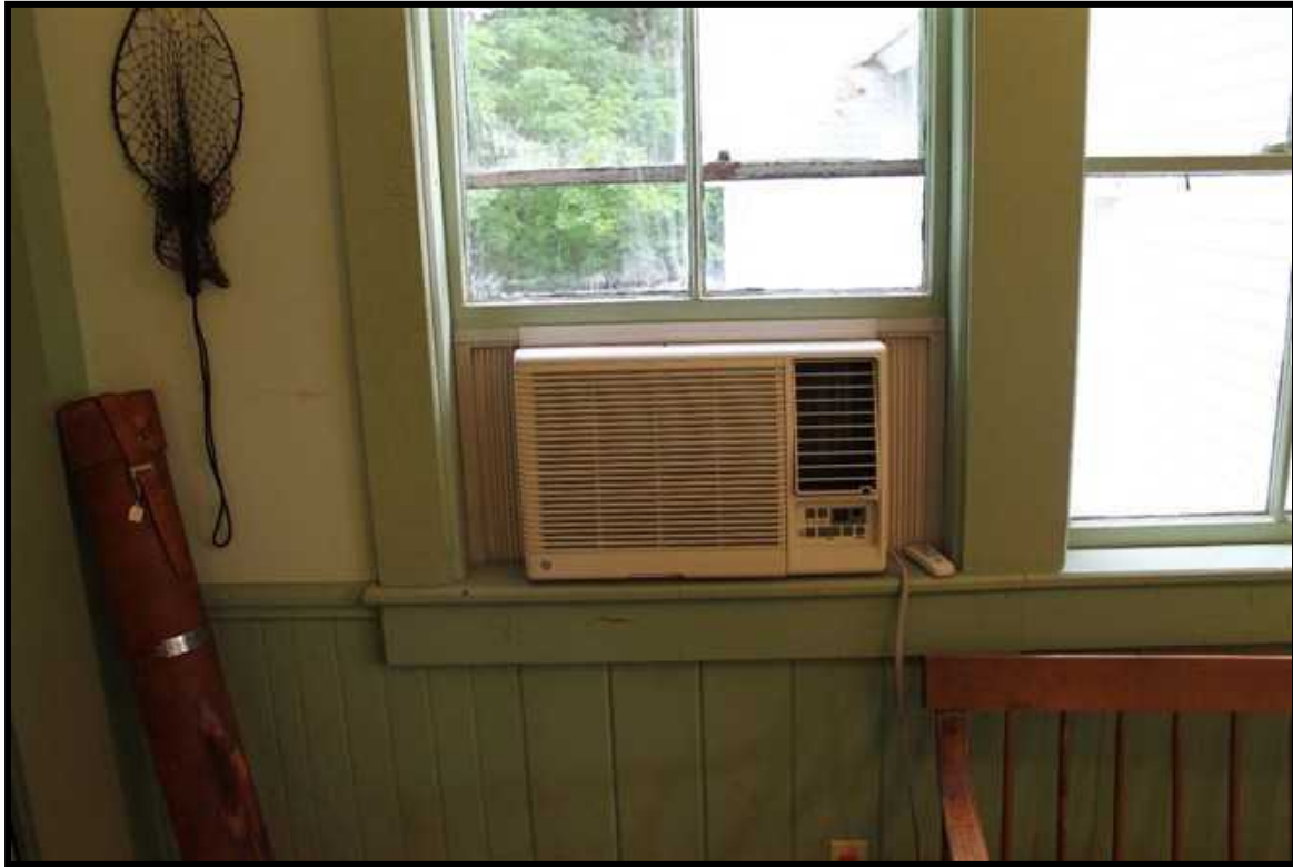
Image Interior Detail 009 – Window Air Conditioner Installed.
