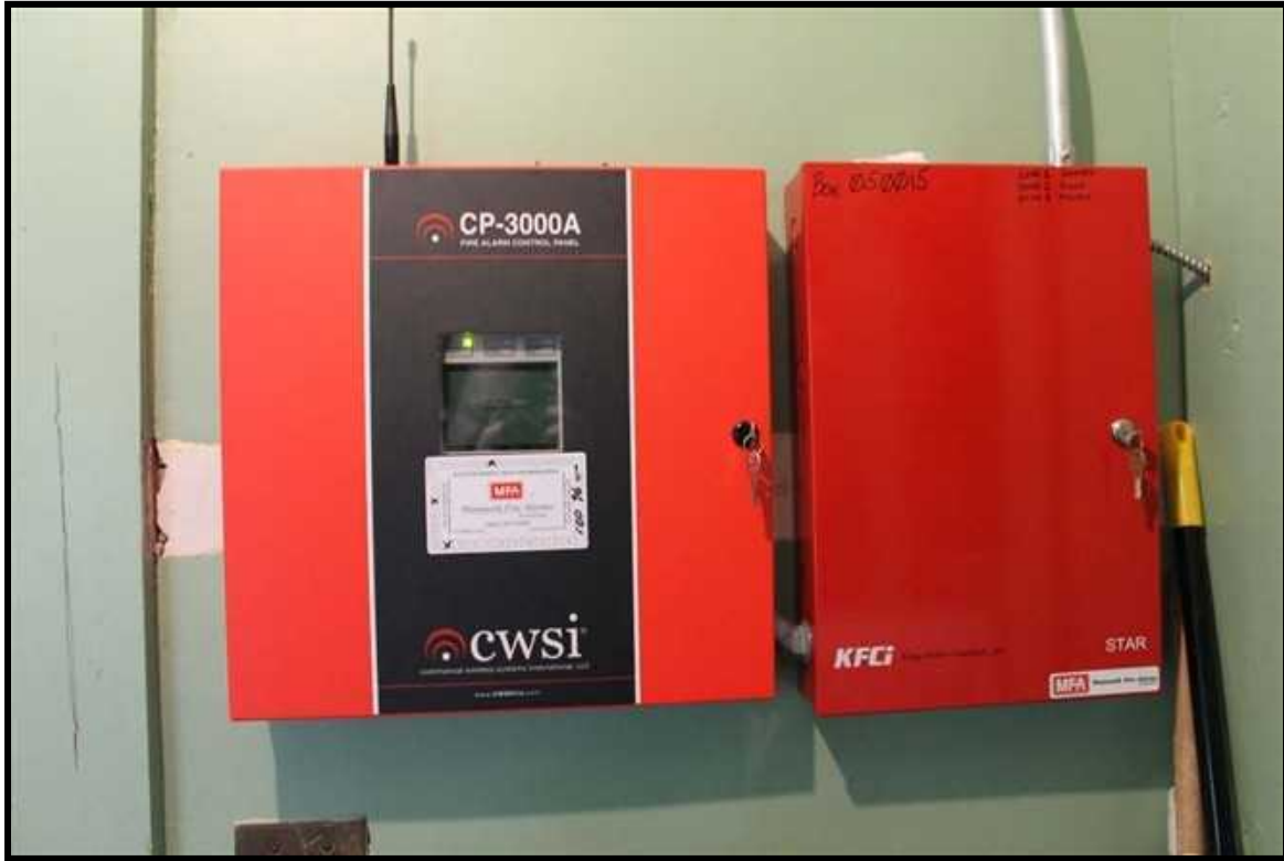
Image Interior Detail 011 – Existing Alarm Panel
