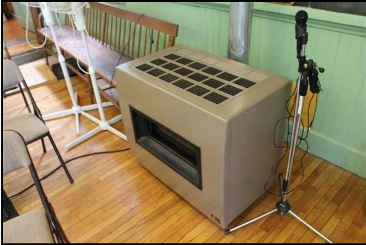
Image Interior Detail 003 – Furnace in 1886 Schoolhouse
