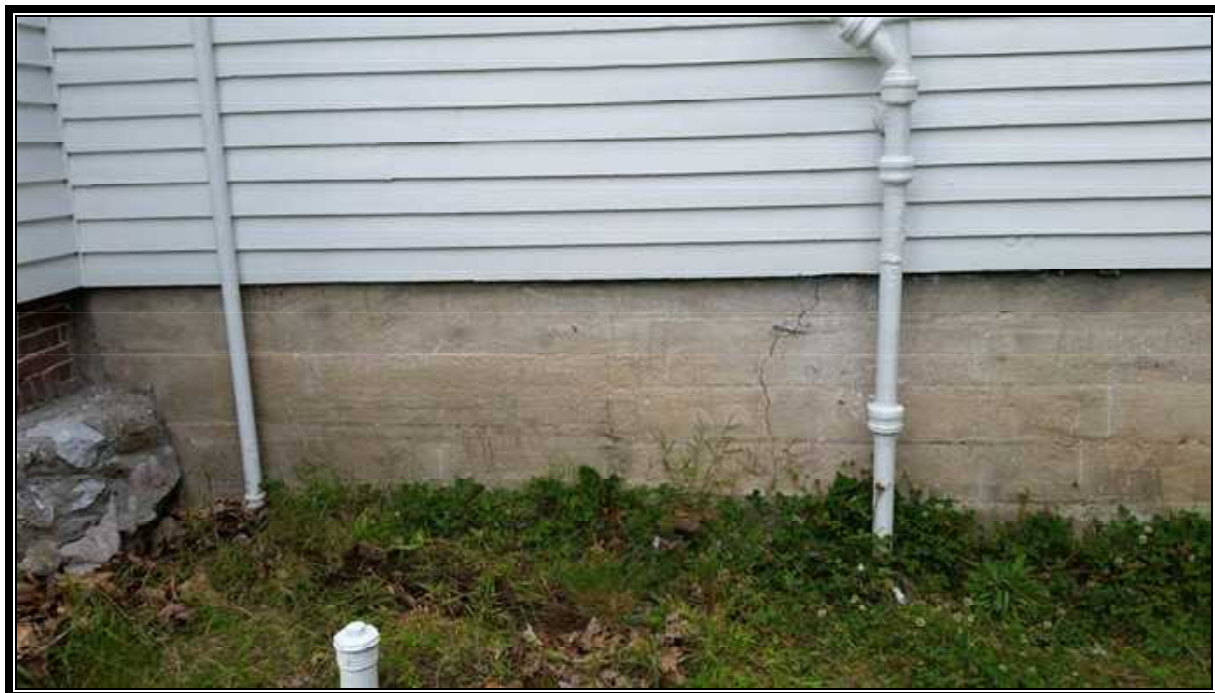
Photo 6: Minor crack in concrete wall.
