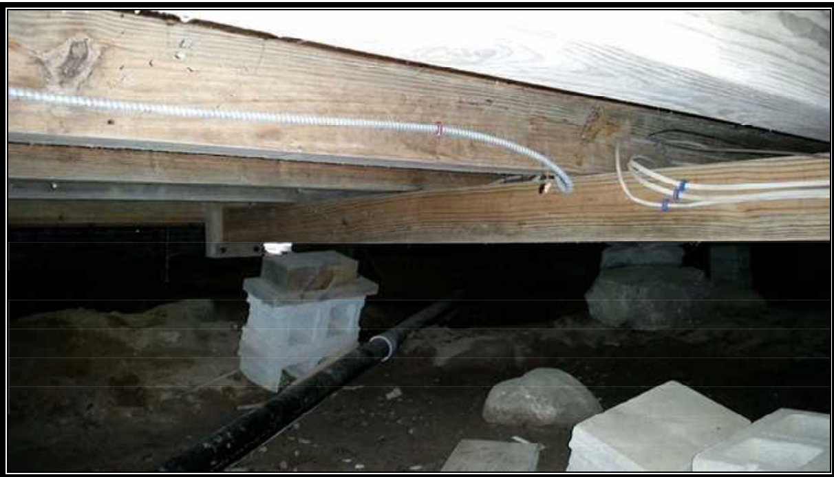
Photo 4: CMU pier not supporting beam.
