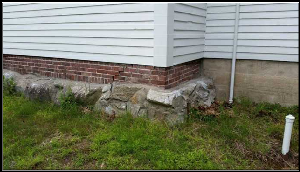
Photo 3: Settling crack at corner of foundation.
